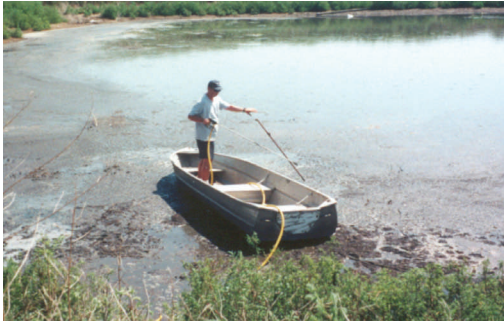
PitCharger being injected into heavy sludge in the earthen basins of an older facility acquired by Zoltenkos.
